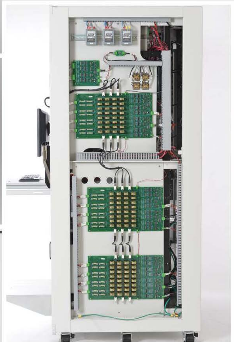
Side view with Left Extension Open allowing easy access to all of the Switching Matrix Cards, HF Relays, Power Supplies, Relay Drivers etc
