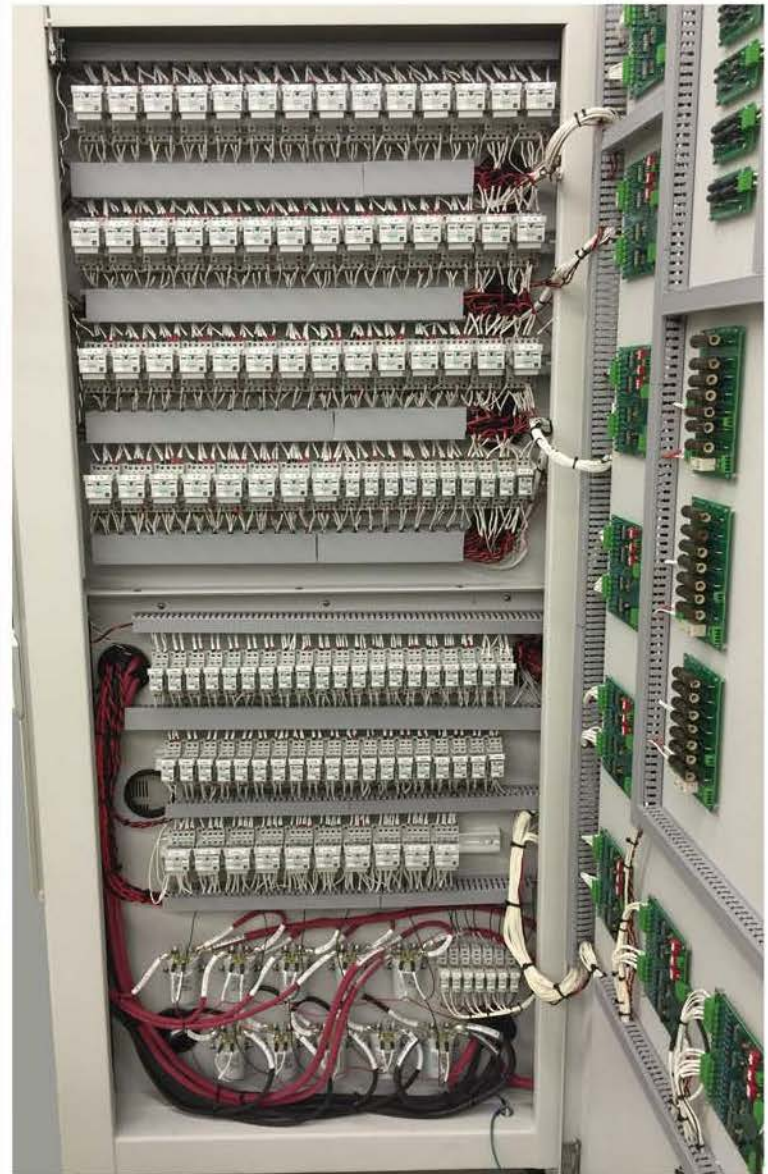
Right-Side Cabinet Extension Open showing over 100 DIN Rail Relays, Relay Drive PCBs, Resistors, High Power Relays, etc.
