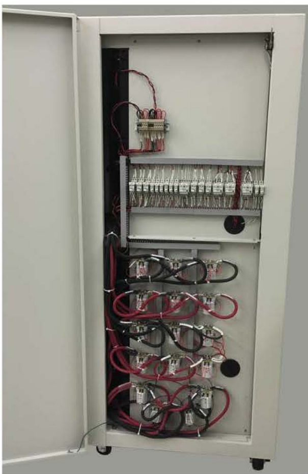
Left-Side Cabinet Extension Open showing High Power Relays, DIN Rail Relays, Terminal Blocks, etc.
